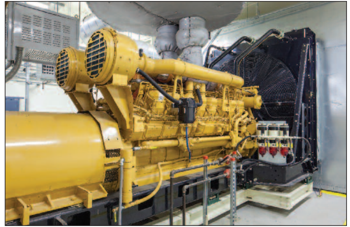
Standby generator rooms need protection and are in most facilities.
